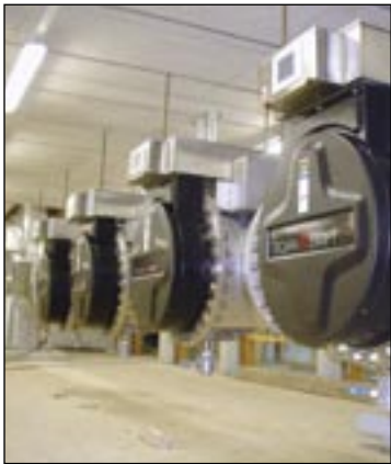
Using a combination of UV light and hydrogen peroxide, the TrojanUVSwift™ECT system provides superior disinfection without producing harmful by-products such as bromate.
