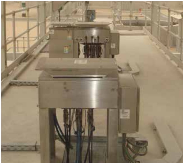
Wastewater disinfection in Alkhor, Qatar – 380 m 3 /hr (2 MGD)
