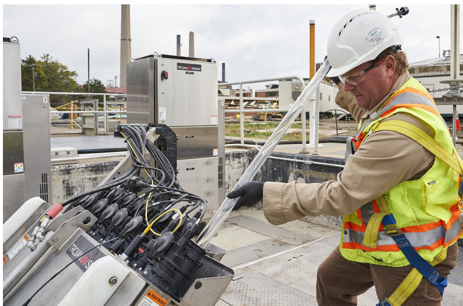
Core components of a wastewater UV system include lamps and drivers, quartz sleeves and the sleeve cleaning system.
