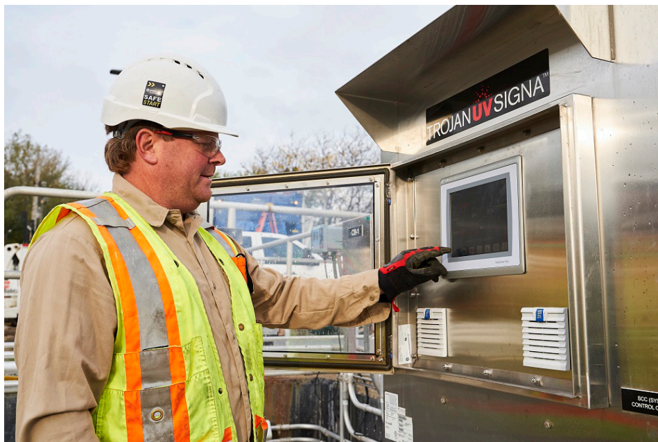
The SCC monitors and controls all UV functions to ensure optimal disinfection performance.
